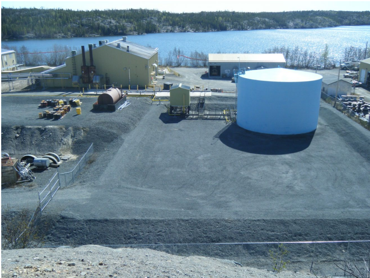
Figure 2: 1,700,000L Fuel Tank in New Berm
