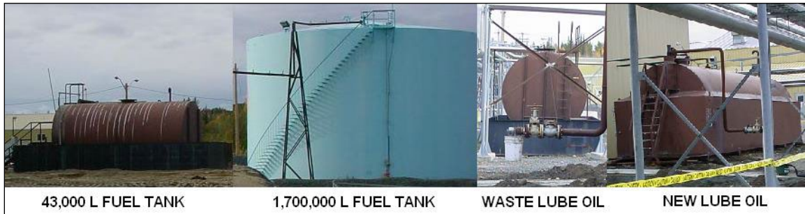
Figure 3: Facility Fuel & Lube Oil Storage (showing old 43,000L fuel tank that has been removed)
