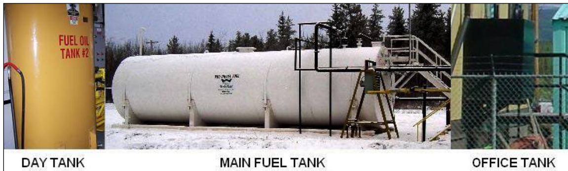
Figure 4: Facility Fuel Storage
