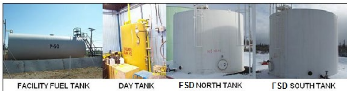
Figure 4: Facility Fuel Storage
