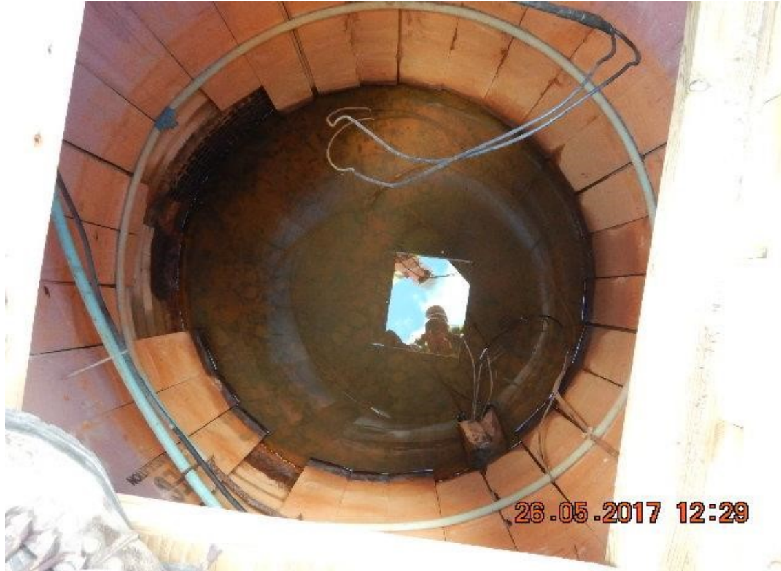
Figure D.5: Snare Rapids Main Dam LB seepage collecting well
