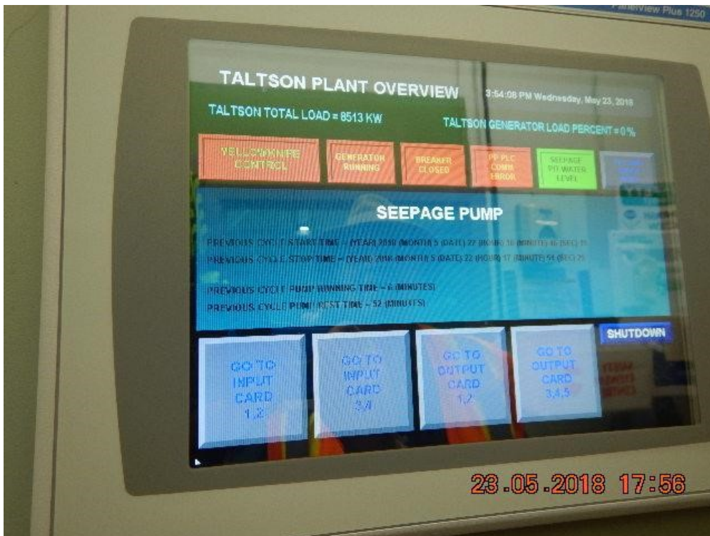
Figure D.38: Taltson seepage monitoring HMI inside the powerhouse
