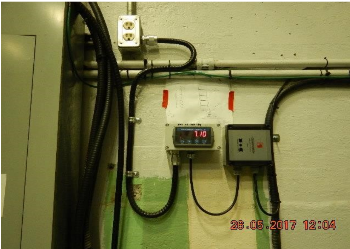
Figure D.4: Snare Rapids seepage monitoring meter (inside the powerhouse)
