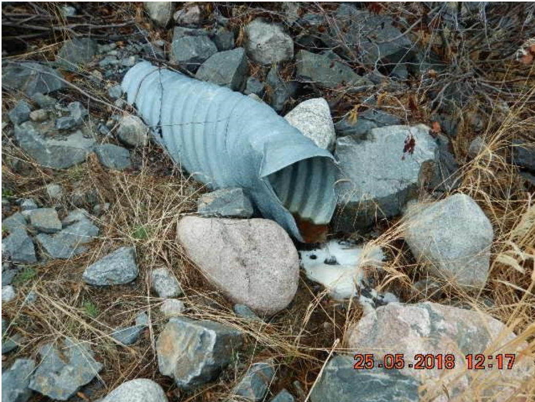
Figure D.25: Snare Forks seepage monitoring at Forks Main Dam Downstream
