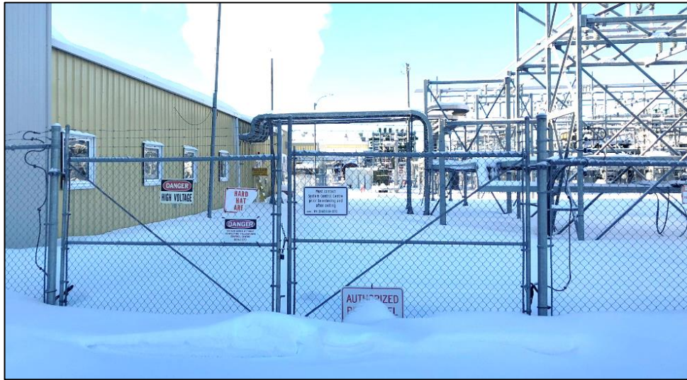
Figure 6: High Voltage Warning Signs
