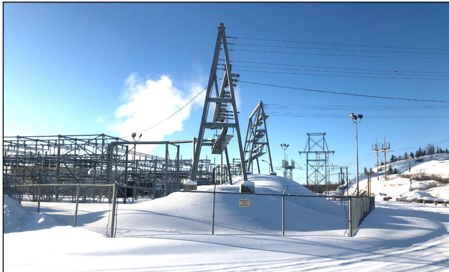
Figure 5: Jackfish Lake Generating Facility
