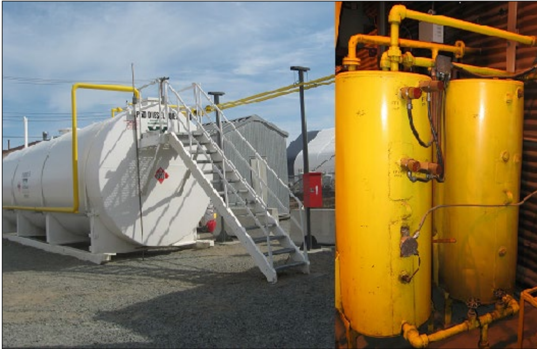
Figure 3: Facility Fuel Storage
