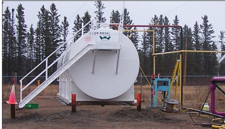
Figure 3: Facility Bulk Fuel Storage
