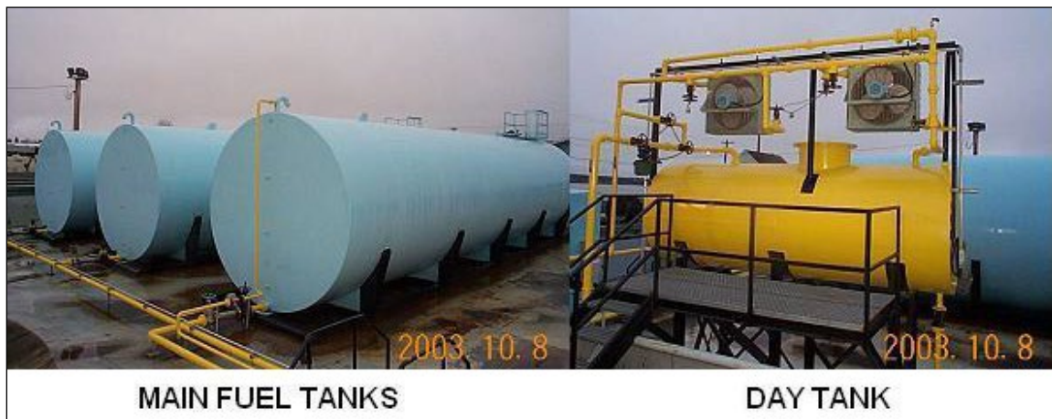
Figure 4: Facility Fuel Storage
