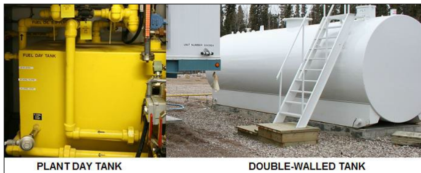
Figure 3: Facility Bulk Fuel Storage
