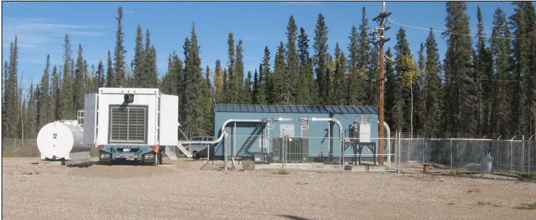
Figure 2: Fort Resolution Power Plant
