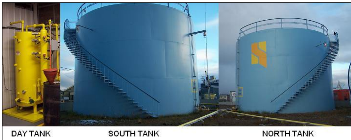
Figure 3: Facility Fuel Storage
