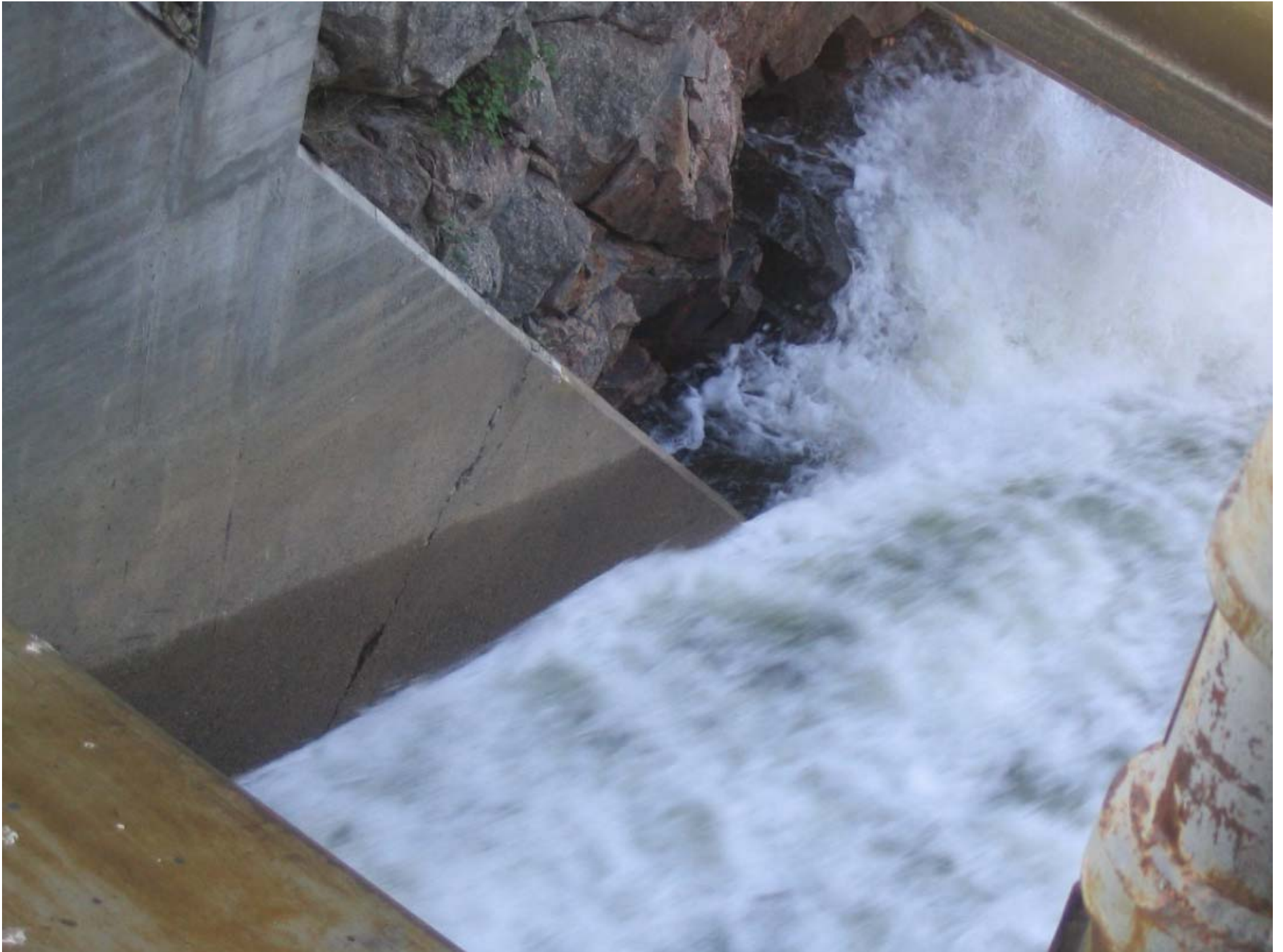
Snare Falls Spillway – Diagonal Cracks on Downstream Pier
