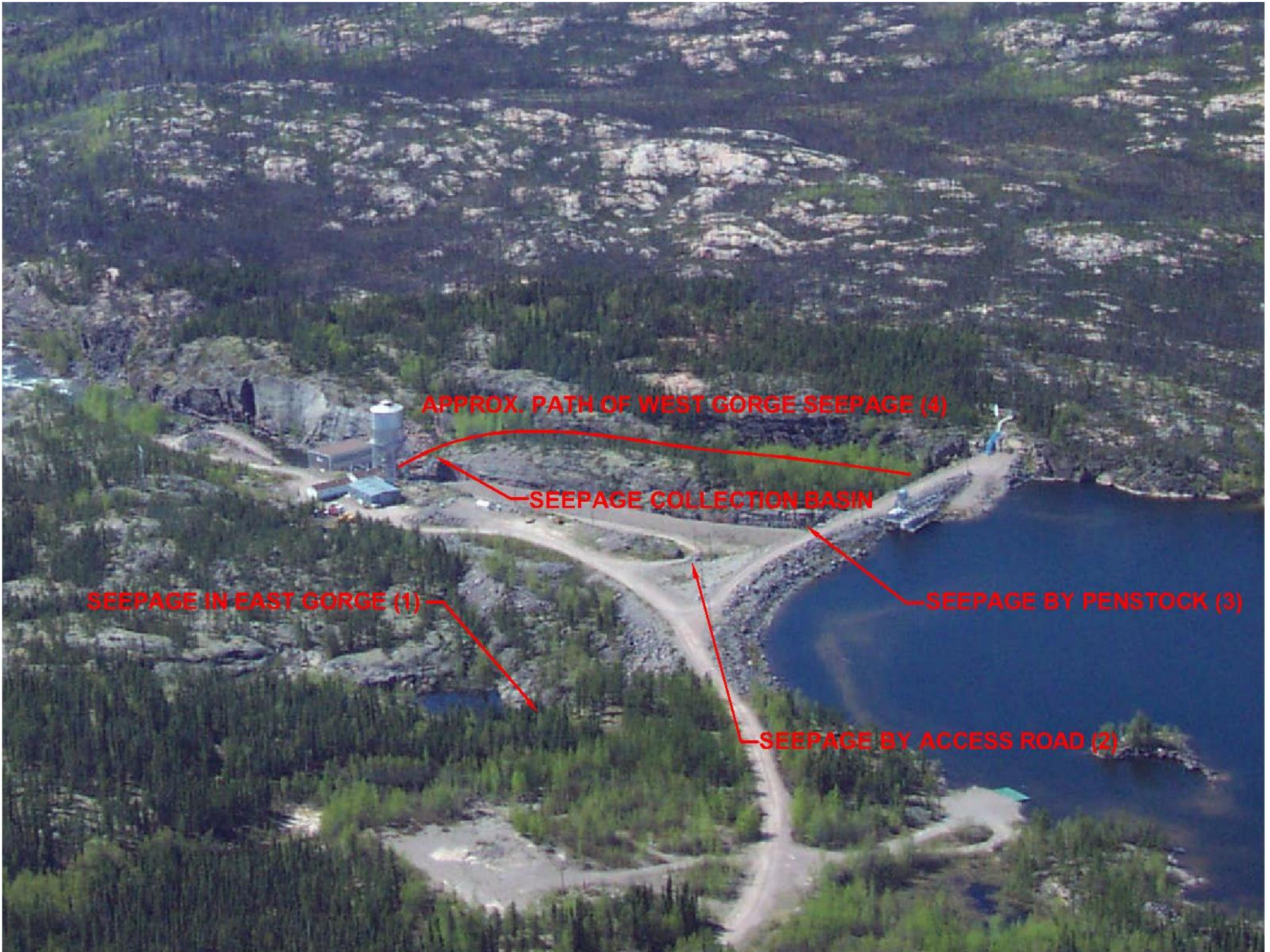
Taltson Dam – Aerial Photo Showing Seepage Locations
