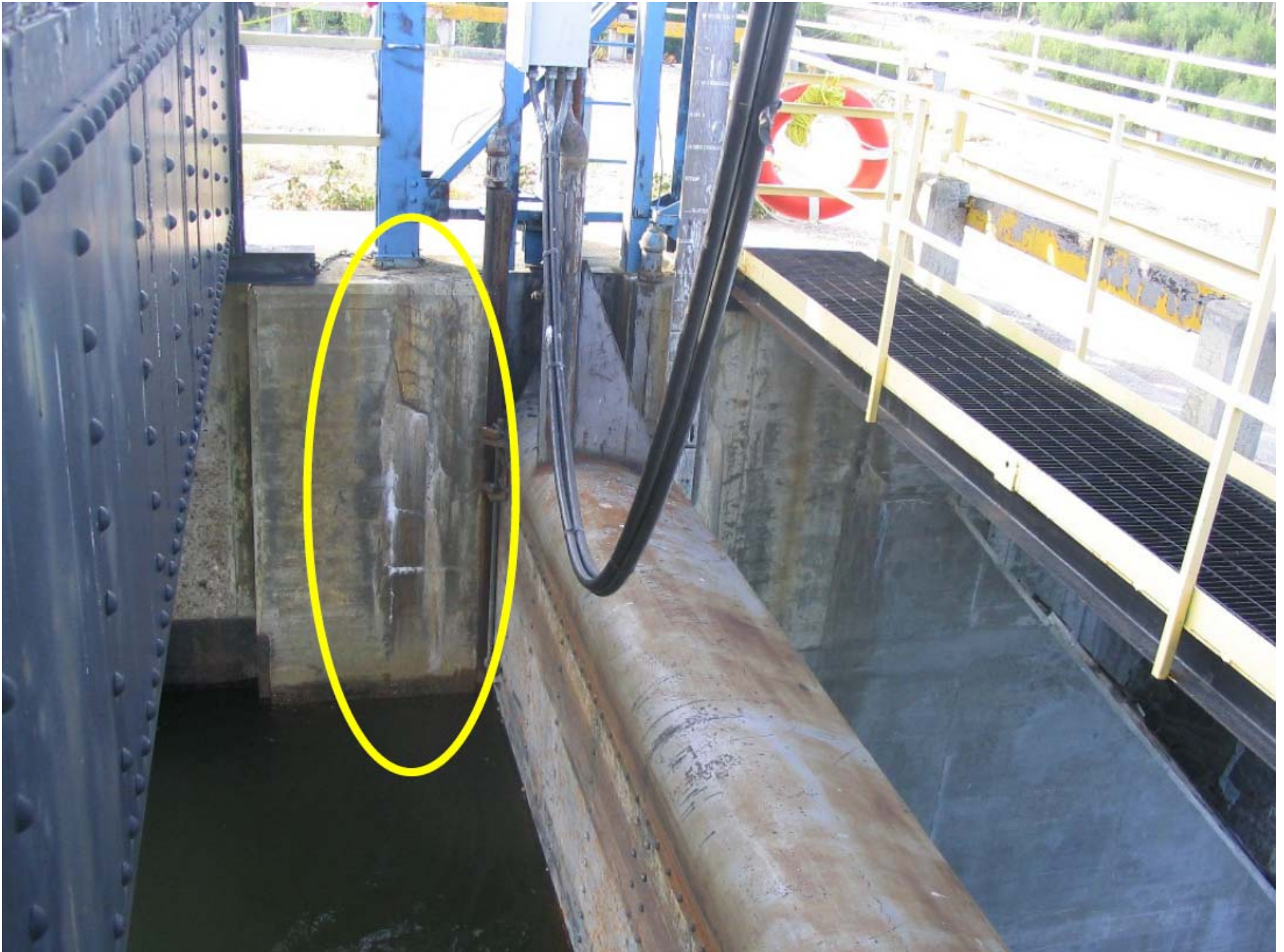
Snare Falls Spillway – Vertical Cracks Adjacent to Gate Guides
