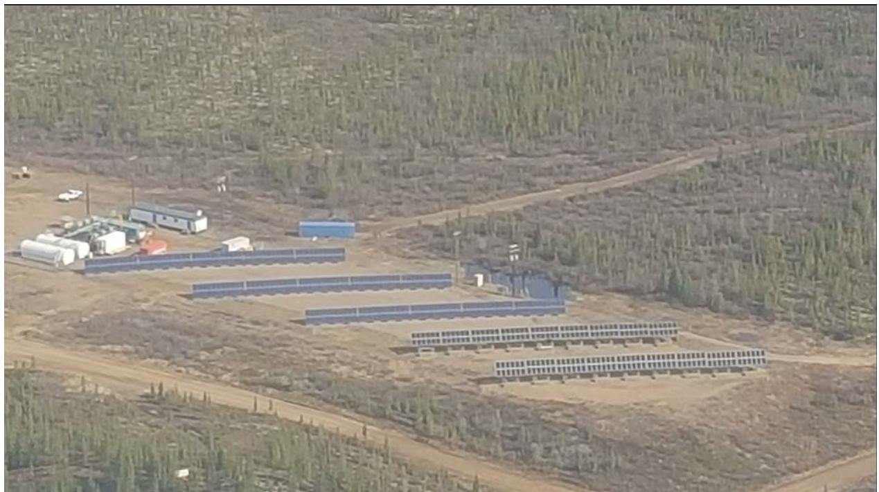
Figure 2: Colville Lake Plant
