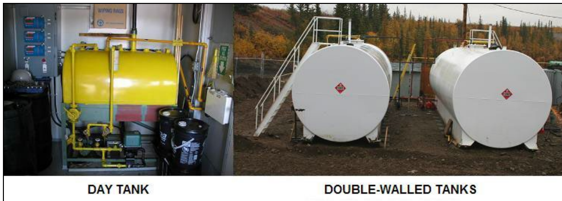
Figure 3: Facility Fuel Storage
