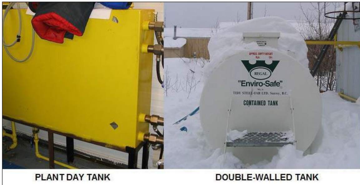
Figure 3: Facility Fuel Storage
