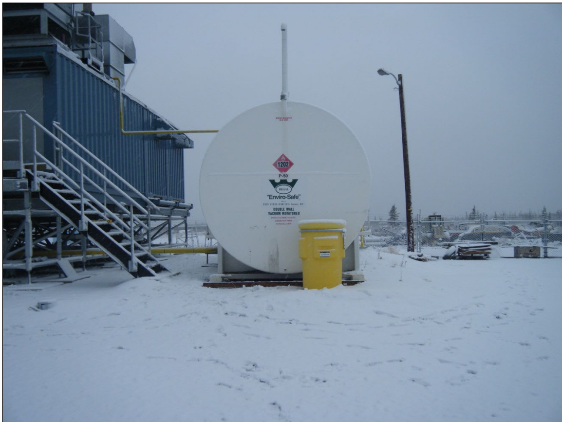
Figure 3: Facility Fuel Storage
